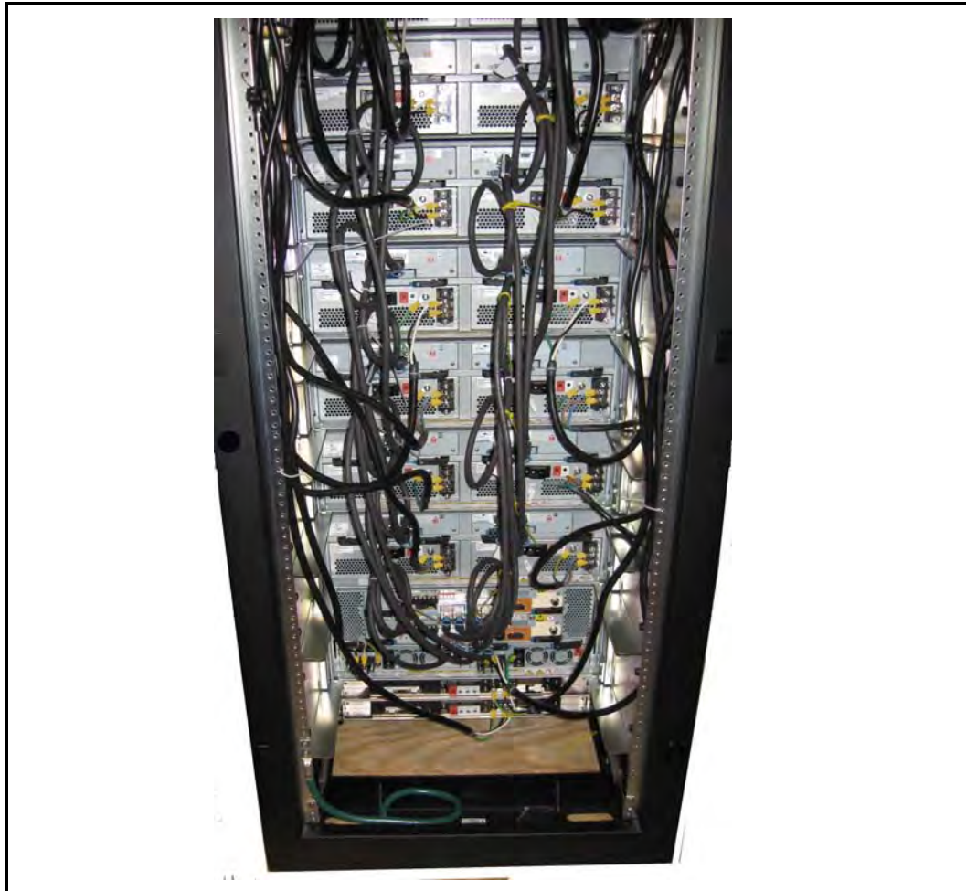
Figure 6-2: Seismic Rack - Rear View
